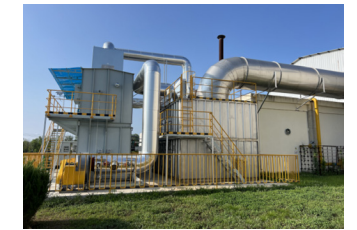
RTO Waste Gas Treatment Equipment
